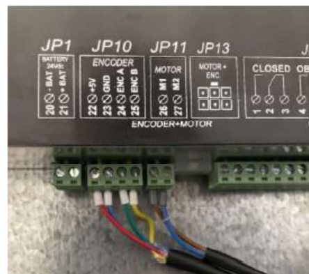
Run new extension cable from the drive to the new motor termination box on top of car
