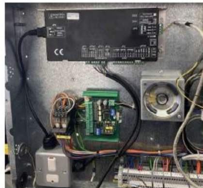
Remove existing drive board and fit new drive and mains spur box
